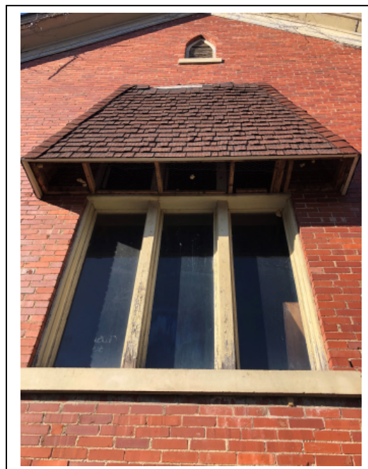
These old awnings on the former UEB Church are inconsistent with the guidelines both because of their material and because they obscure the distinctive shape of the windows.
