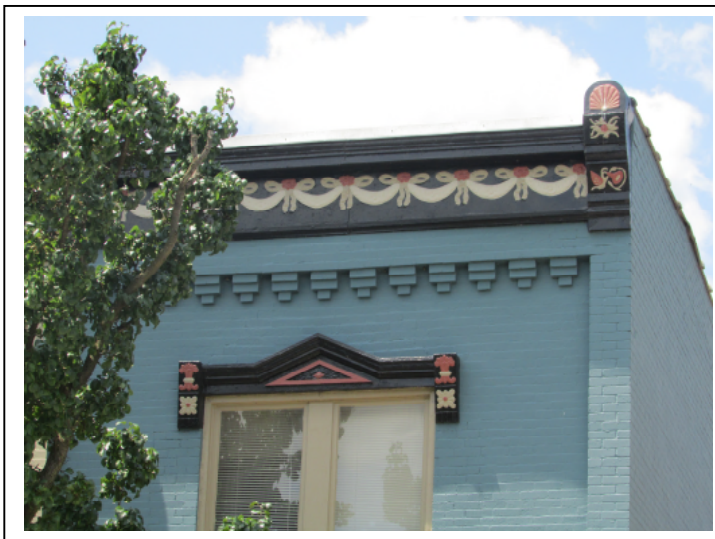
The ornate metal cornice – as well as the decorative brickwork below – is a key architectural feature for this North Capitol Avenue building. The multicolor paint scheme serves to highlight the detail.
