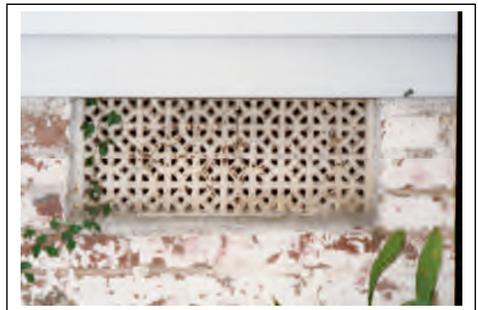
Decorative foundation elements such as cast iron grilles should be preserved and maintained.
